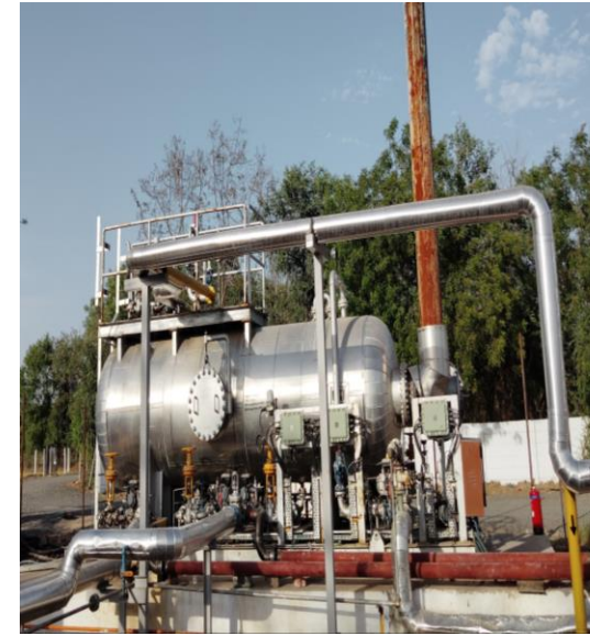
Karjisan Surface Facility Heater Treater area
